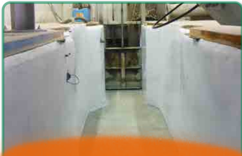
Sewage plants and canals
